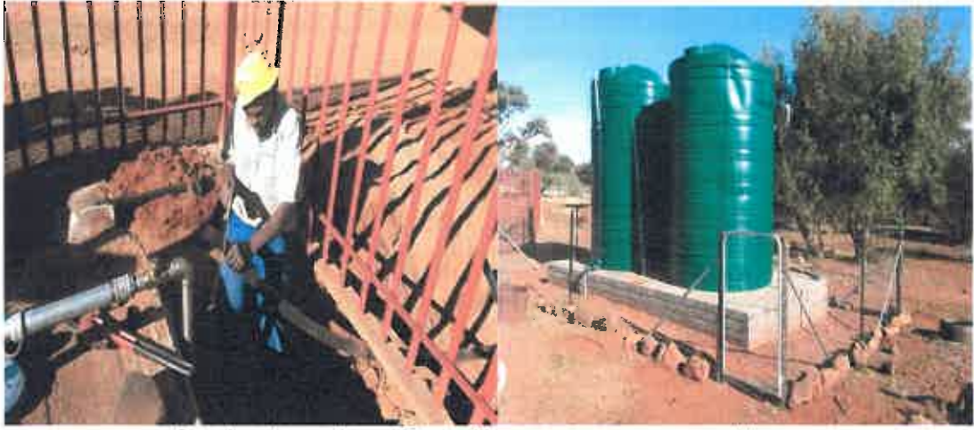
Completion of stock water system at Groenville Commonage at Barkley West, Frances Baard
