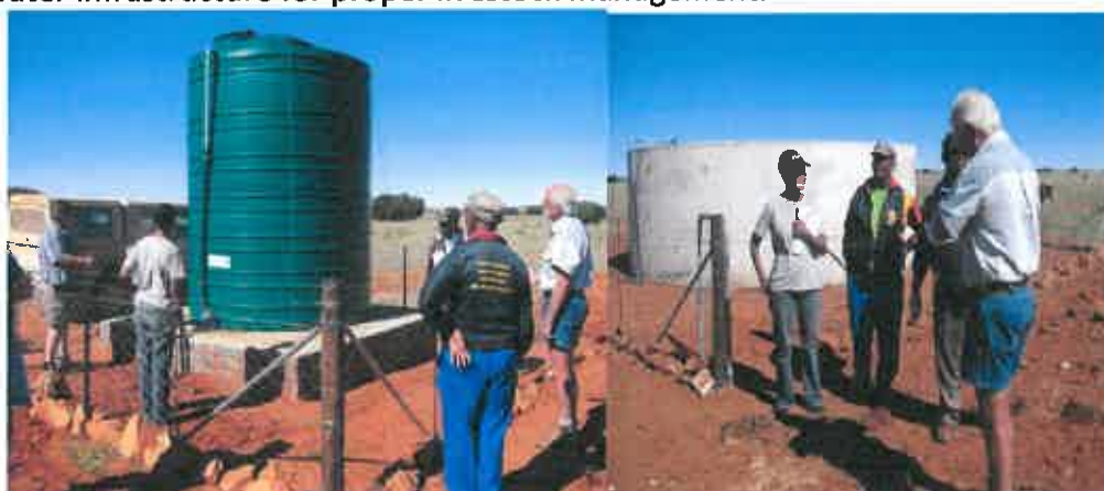
Frances Baard Livestock Project: Completion of stock water system at Waterfall Commonage at Ritchie
